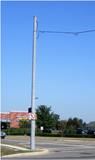
Non-Ornamental Municipal Service Pole
